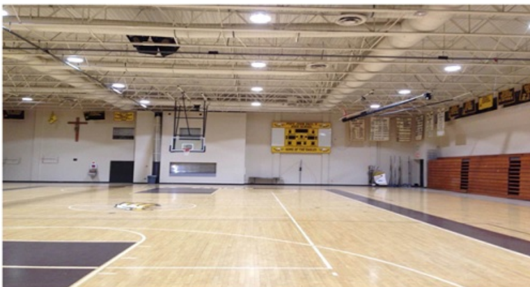
(In October of 2015, 24 new LED High Bay fixtures were installed at St. John Paul II High School in Boca Raton, Florida)
